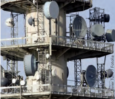
Telecom - Data infrastructure
